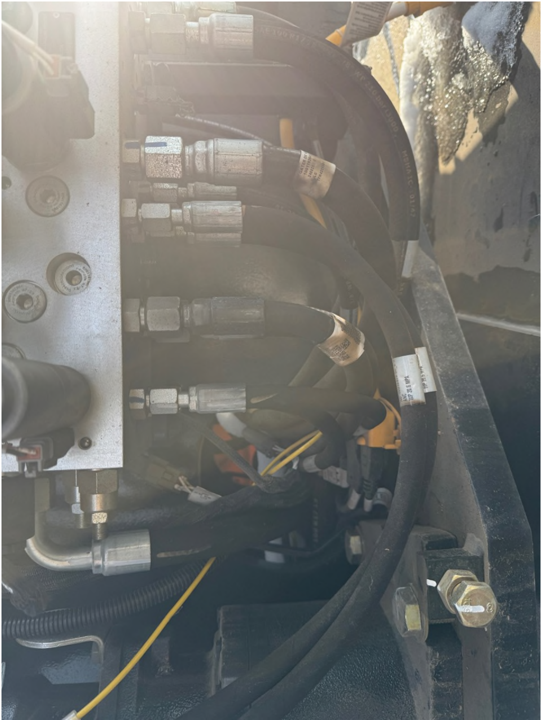
Interior view beneath the side panels on each side of the unit showing the motor, hydraulics, and electrical controls.
