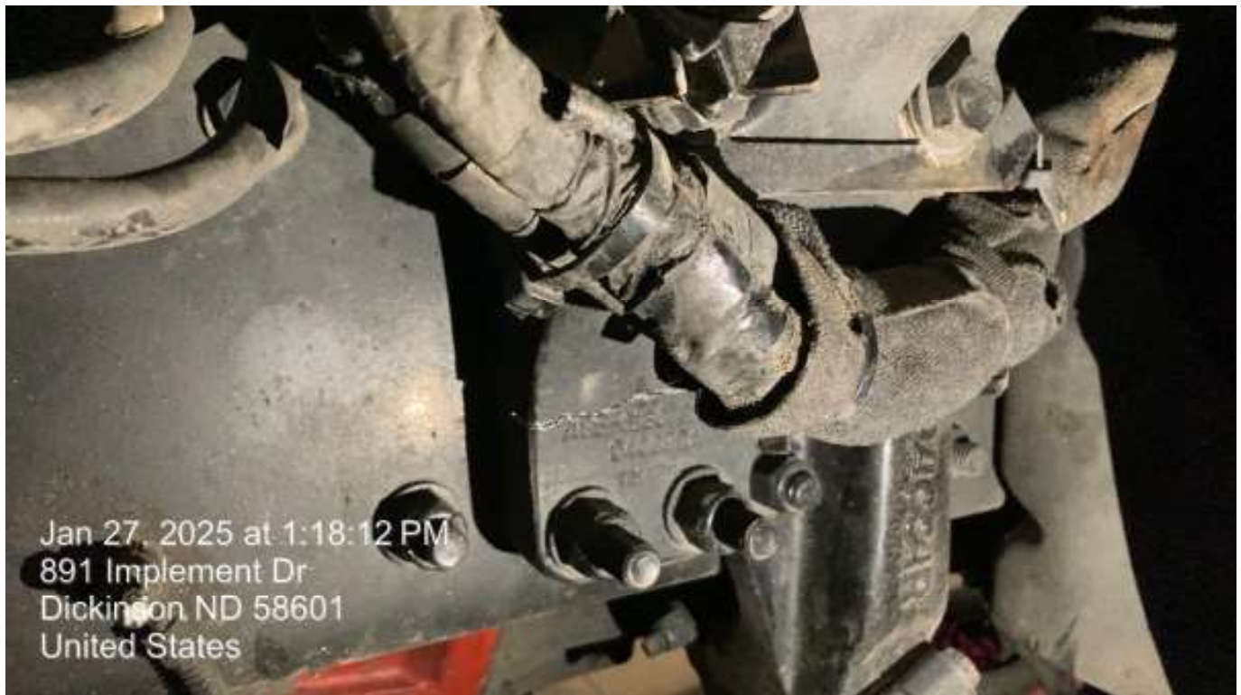
bolted support to frame is cracked
