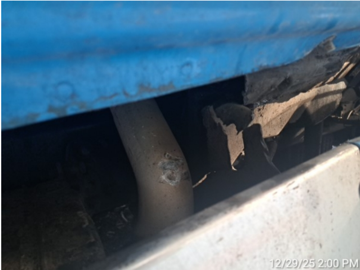
RT SIDE DAMAGE
